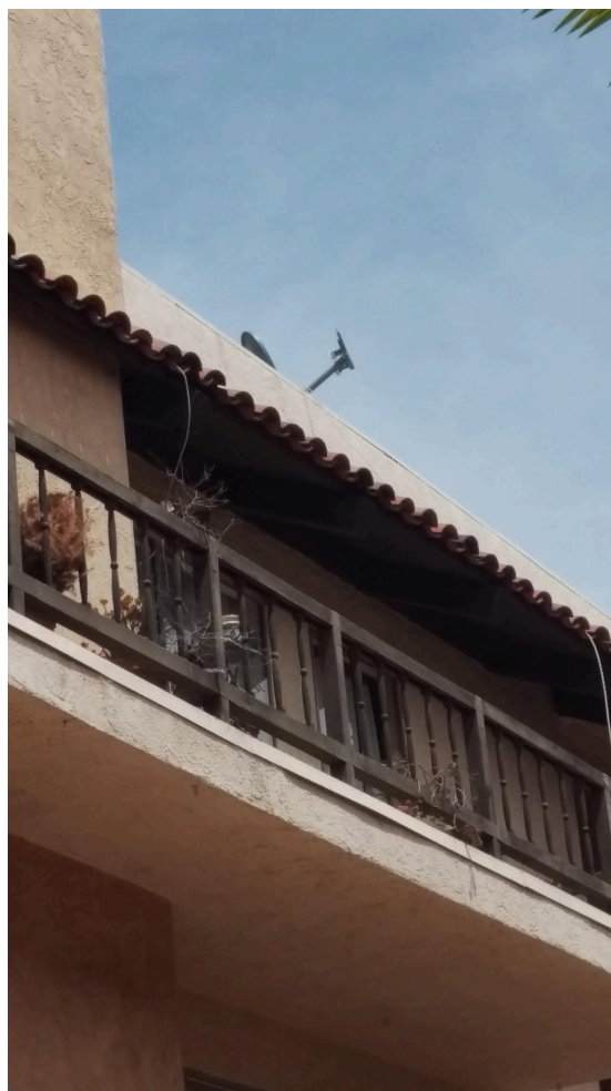
Mounted on front parapet & bad cabling
