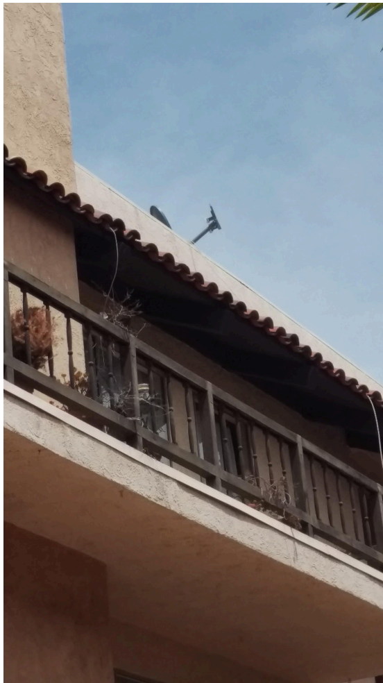
Mounted on front parapet & too close to the roof seal line
