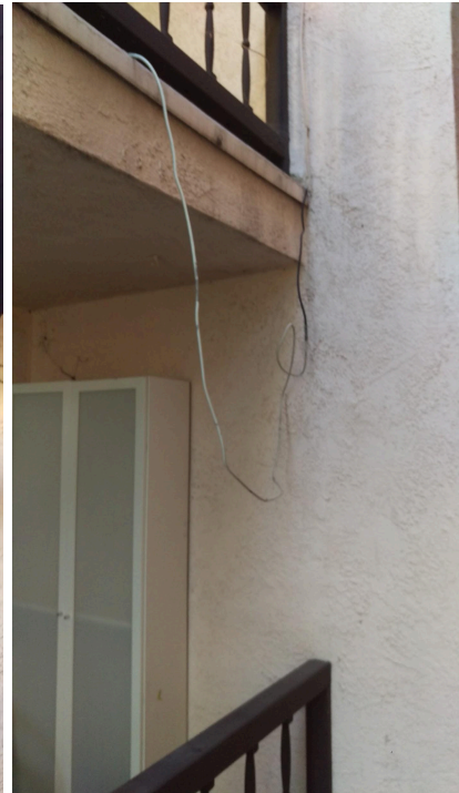
The wrong way
